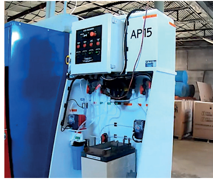
The Mech-Chem AP-15 system used by River Street to filter sulfuric acid
