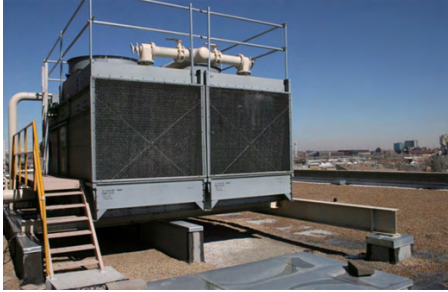
Photo: Denver Water, http://www.denverwater.org/conservation/incentiveprograms/indoorcommercial/coolingtower/
