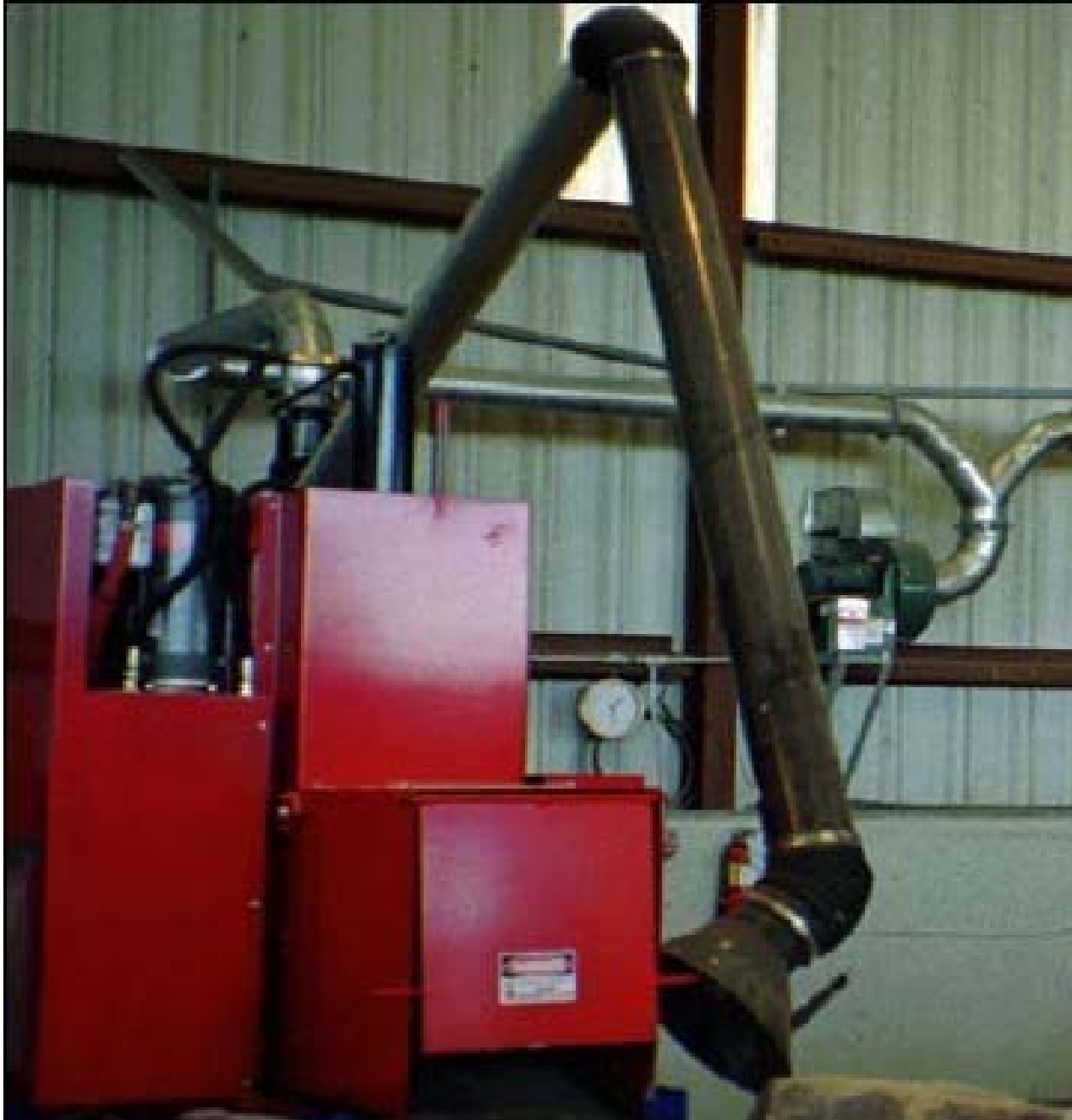
HHV Spot Ventilation at Cowlitz County
