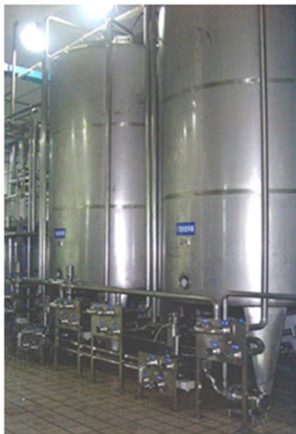
300 Gallon SS Tank @ 70°C
