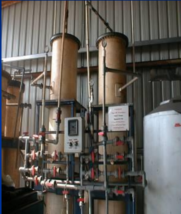
Ion Exchange Unit
