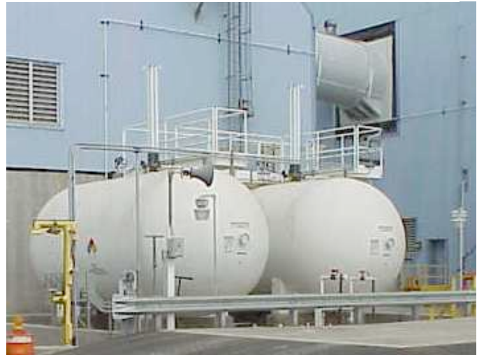
Figure 1: Anhydrous Ammonia Tanks
