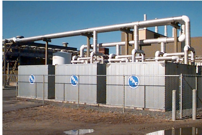
Figure 1: Building 11 Ice Storage System
