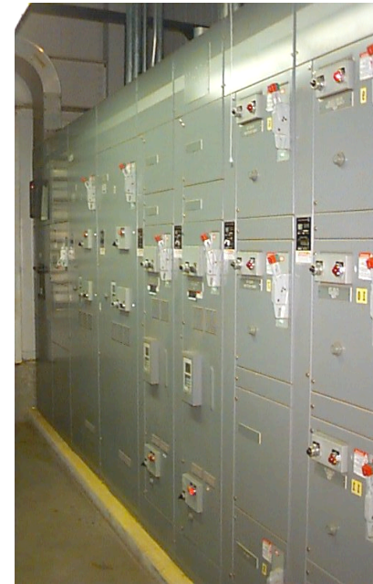
Figure 3: Variable Frequency Drives
