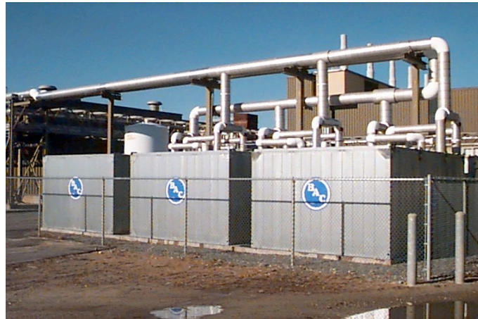
Figure 1: Building 11 Ice Storage System
