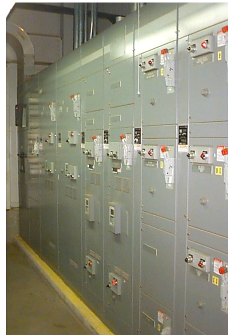
Figure 4: Variable Frequency Drives
