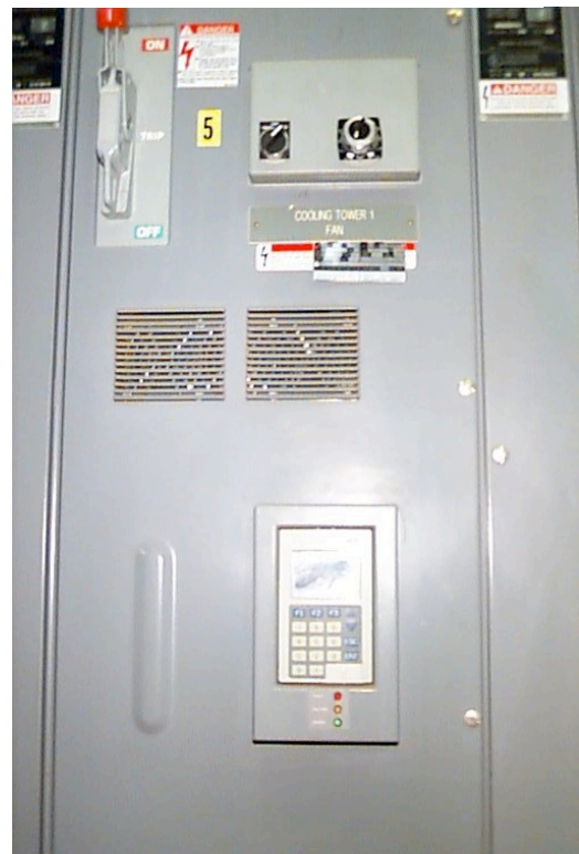
Figure 1: Cooling Tower VFD Panel
