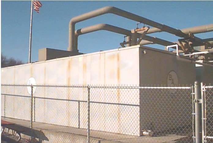
Figure 3: Building 12 Ice Storage System
