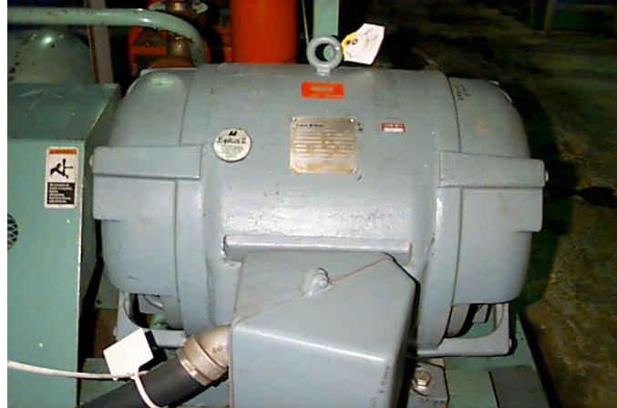
Figure 1: High Efficiency Compressor Motor
