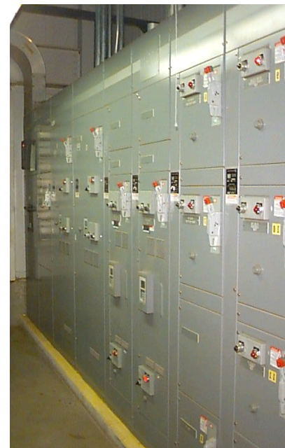
Figure 3: Variable Frequency Drives
