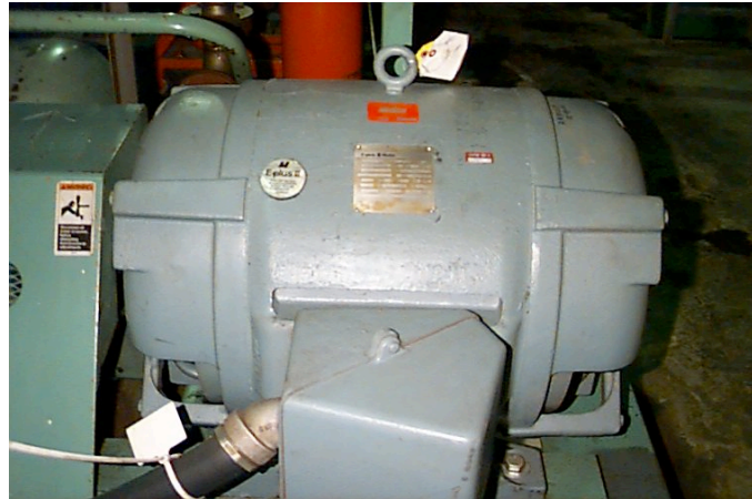
Figure 1: High Efficiency Compressor Motor
