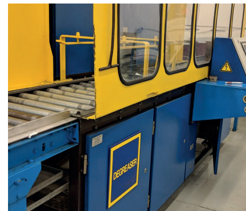
The old vacuum degreaser held 2,000 pounds of perchloroethylene.
