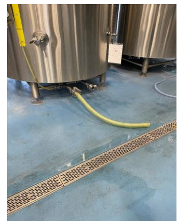
Tank discharge pipe to drain
