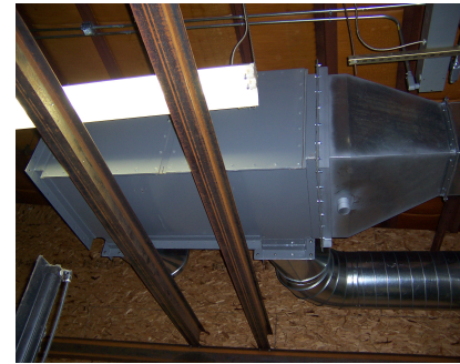
Delaware Valley's Second Heat Exchanger
