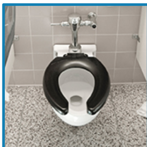
Flushometer Valve Toilets
