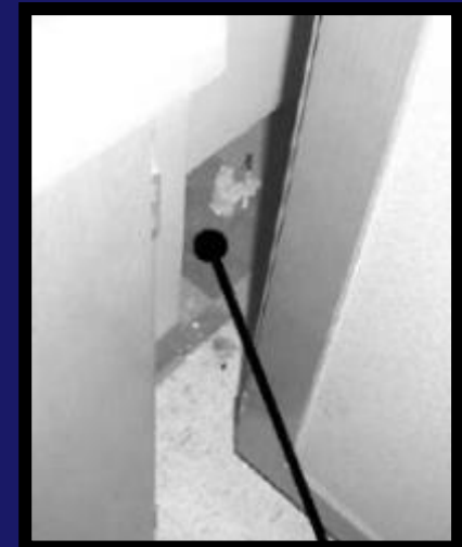
Shelves in classroom built around exhaust cubby obstructing airflow
